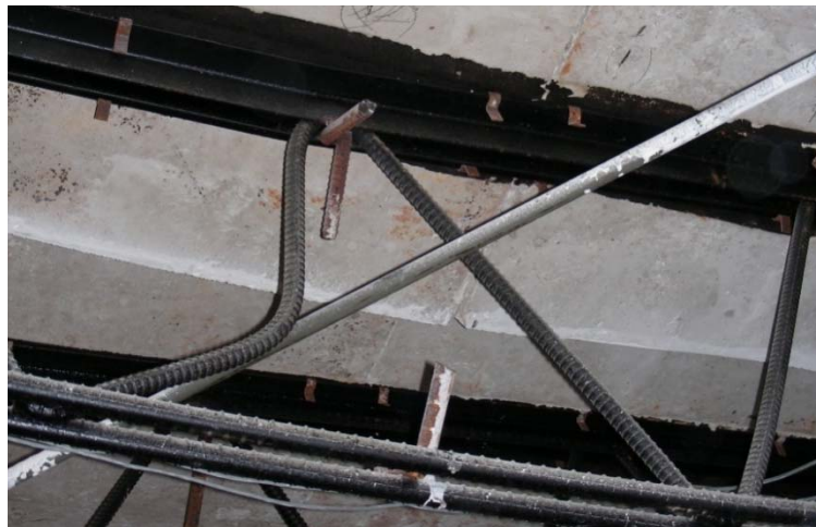
Figure 79 – Diagonal Bar Buckling: Specimen No.2
