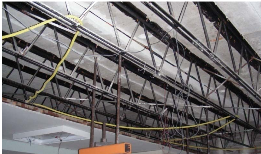
Figure 73-Failure Mode: Yielding Bottom Chord (Specimen no.1)
