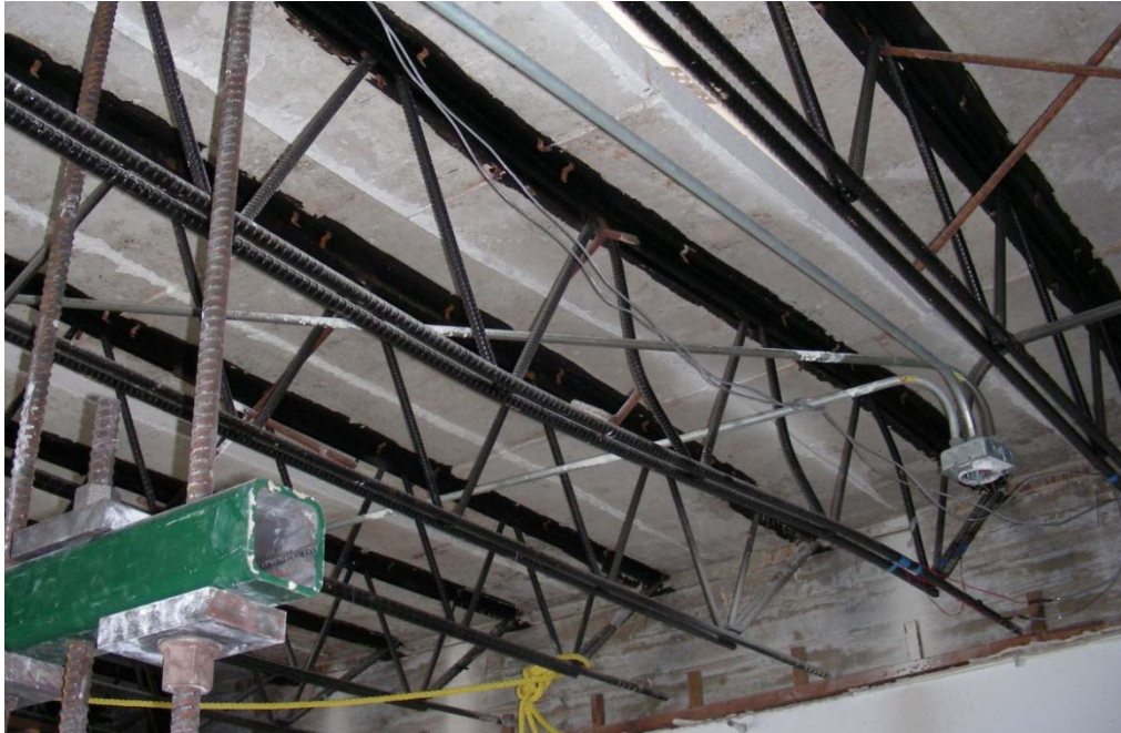
Figure 80 – Buckling Failure: Specimen No.2
